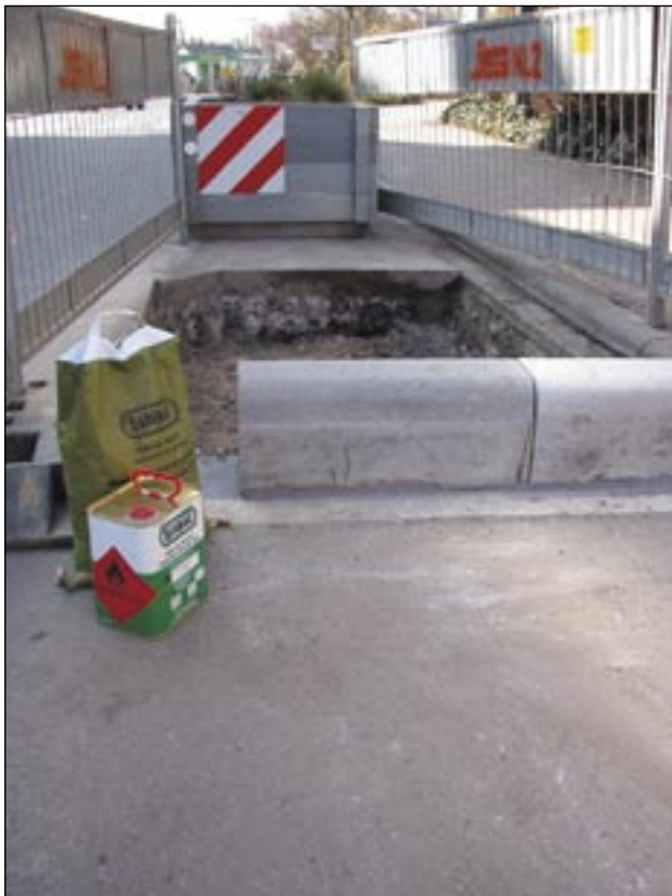
Ladenburg, Schriesheimer street: Building a flower bed with kerb bricks stuck to the asphalt with SILIKAL® Mortar R 17
